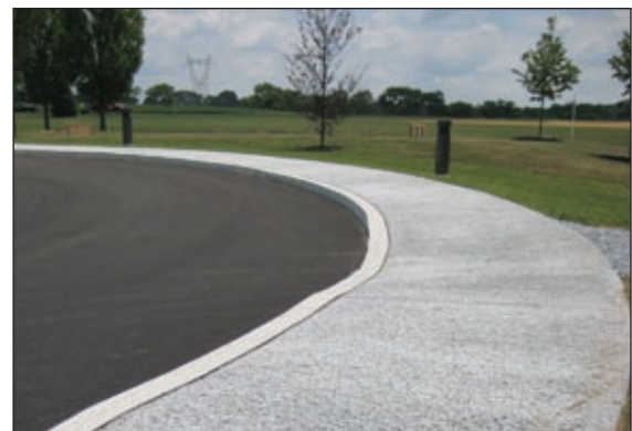
Pervious sidewalks like these at Warwick Township's municipal office help reduce storm water runoff by allowing rainwater to be absorbed into the ground.
