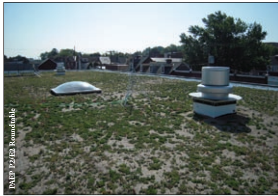
Technical assistance provided by the Lancaster County Planning Commission has helped spur an interest in “green roof” building in the City of Lancaster.
